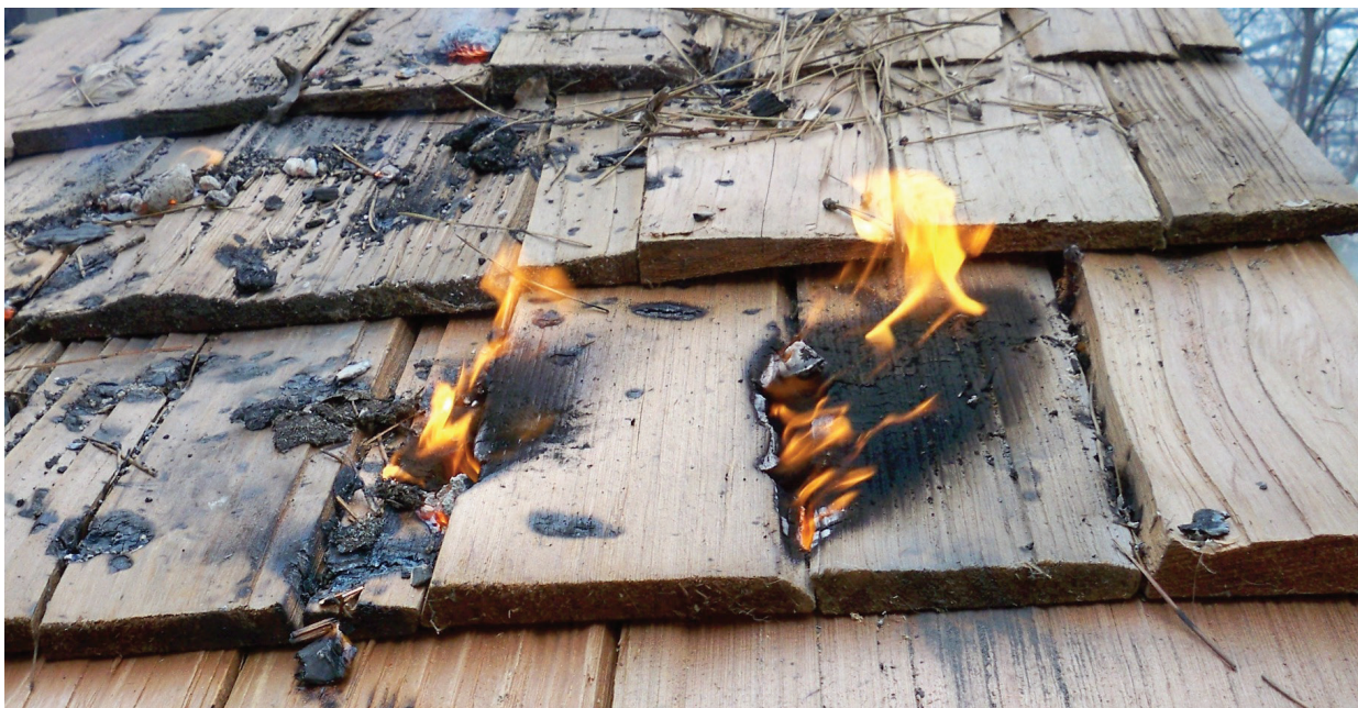
Homes with wood-shake or shingle roofs are much more likely to be destroyed during a wildfire than homes with fire-resistant roofs. Consider replacing wood-shake or shingle roofs with a Class-A fire-resistant type: composition, metal or tile. Photo courtesy http://www.livingwithfire.info
