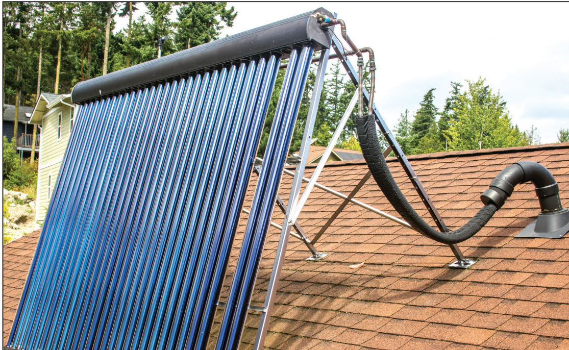
Each solar tube is surrounded on the outside by a transparent layer of glass. Photo by Chris McDaniel
